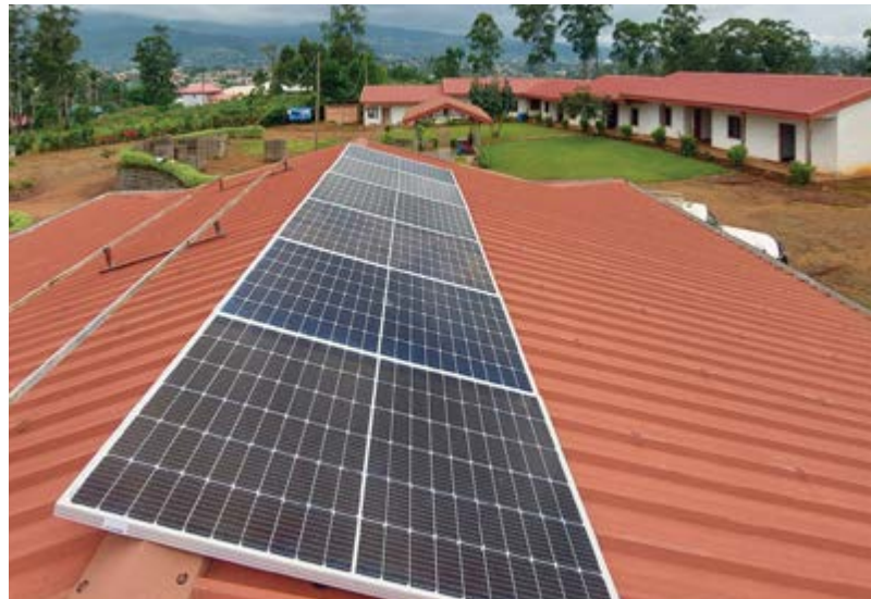
The new solar panels on CABTAL's roof
